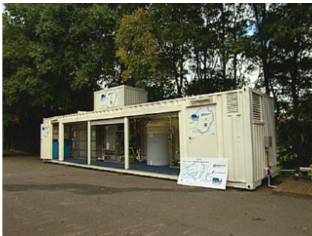
The water recycling plant and irrigation system used in the King’s Domain Gardens in Melbourne, 2002.
